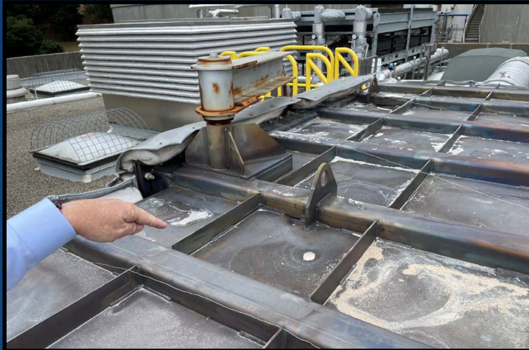
Overheated Emissions Treatment System
