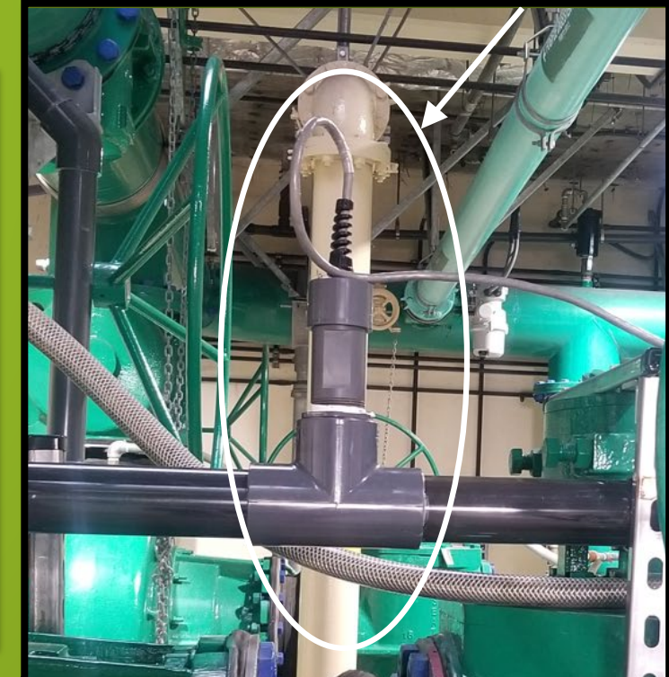
Sentry probes installed at digester recirculation pumps
