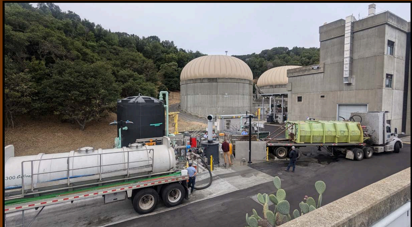
FOG delivery from SRC, 6300 gallons (left), and tested City of Sunnyvale food slurry delivery (5000 gallons, right) in September 2024
